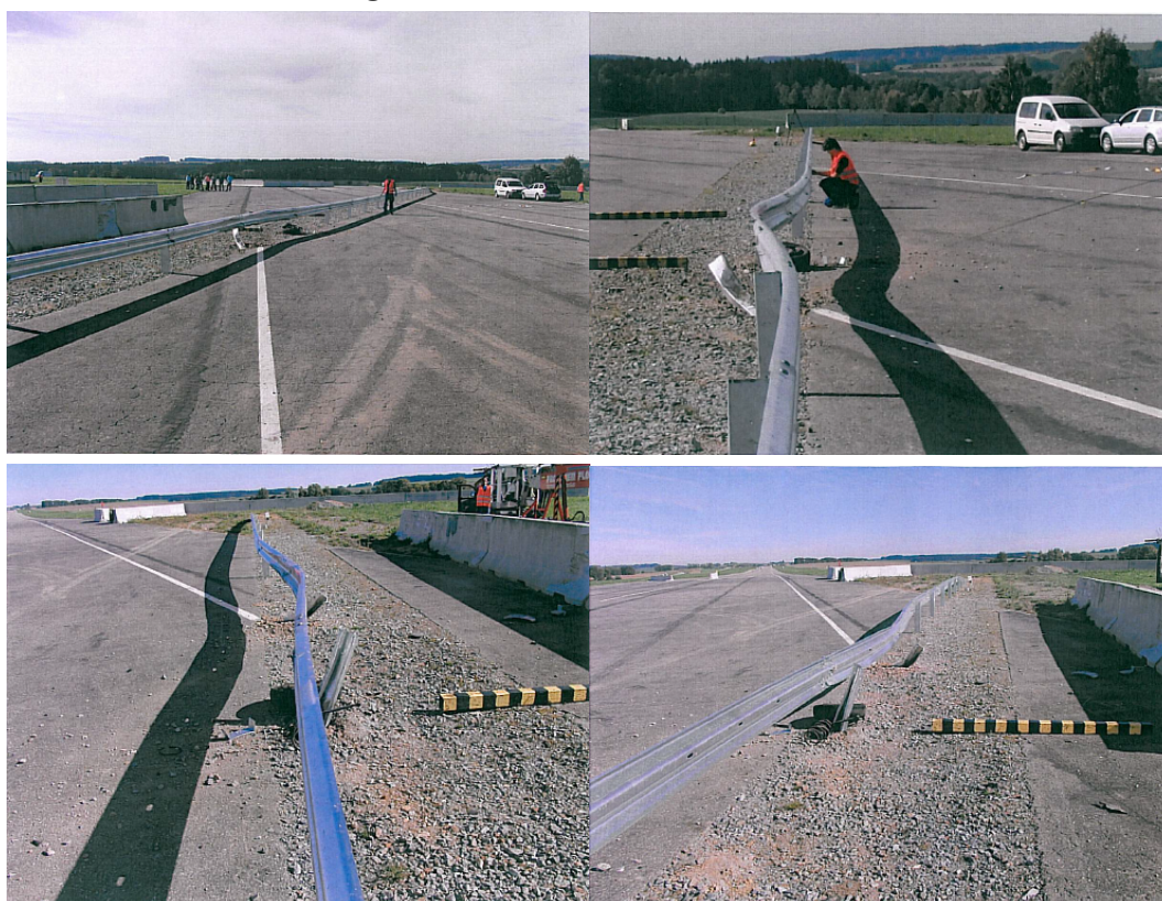
Figure 10: Damage to a crash barrier after impact
