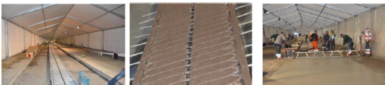
Figure 6. Construction of the concrete test section and details of the induction loops
