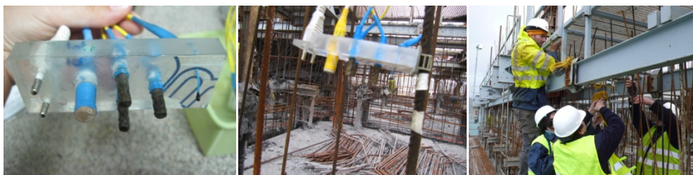
Figure 5: Installation of corrosion electrodes attached to the reinforcing bars of the caisson
